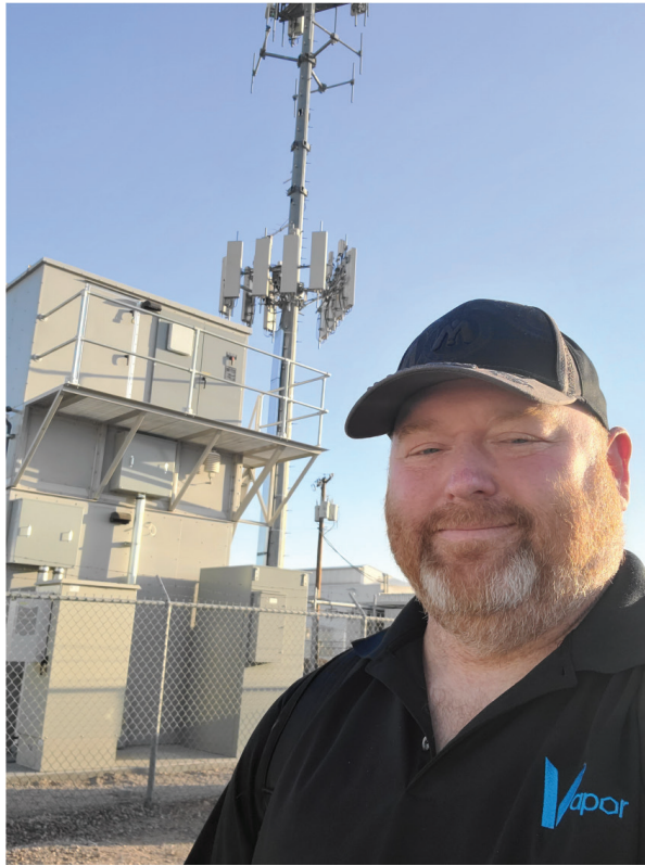
Image: Frank Basso, EVP of Operations at Vapor IO, stands near a newly installed VEM-180 unit.
